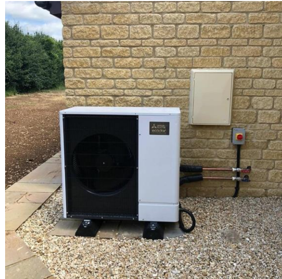
Air source heat pump
